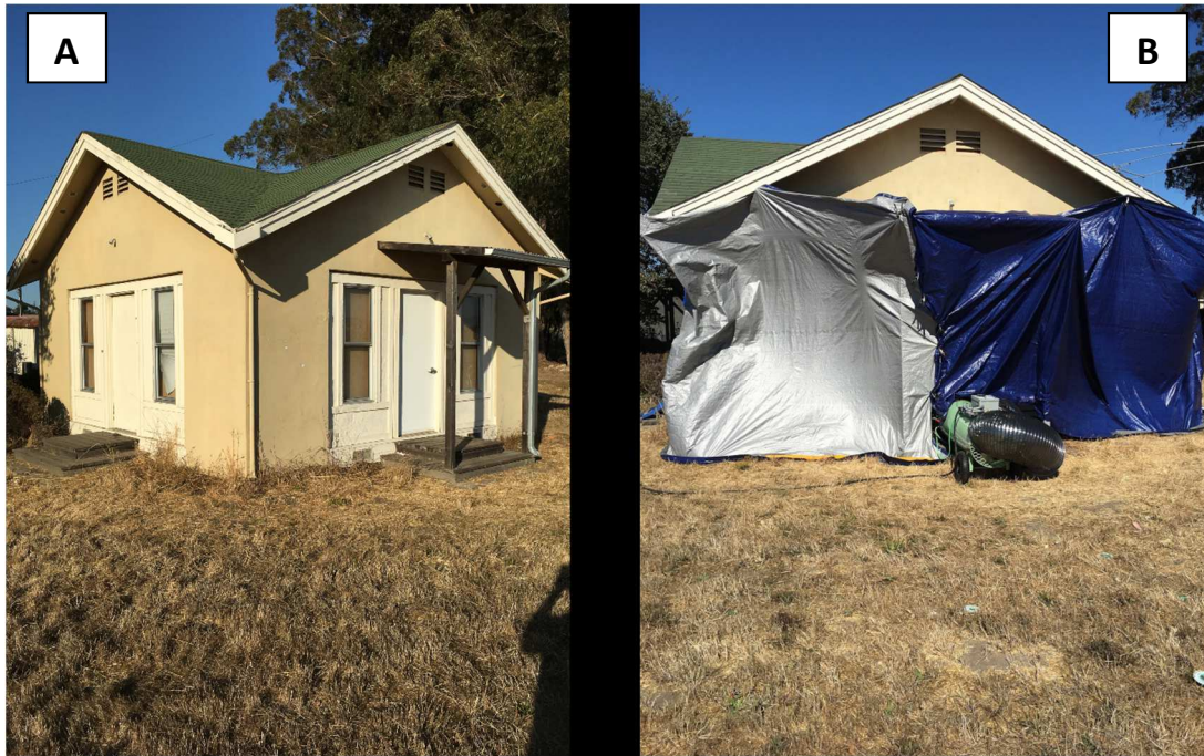
Fig. 3.2. “Villa Termiti”, the experimental structure used in the current study. (A) The south- and west-facing walls of the test structure before beginning treatment. (B) The south wall of the structure during the heat treatment, showing tarpaulins and a heater.
