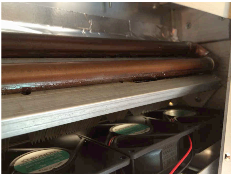
Fig. 3.4: Fans and heat exchanger at the top of the unit.
