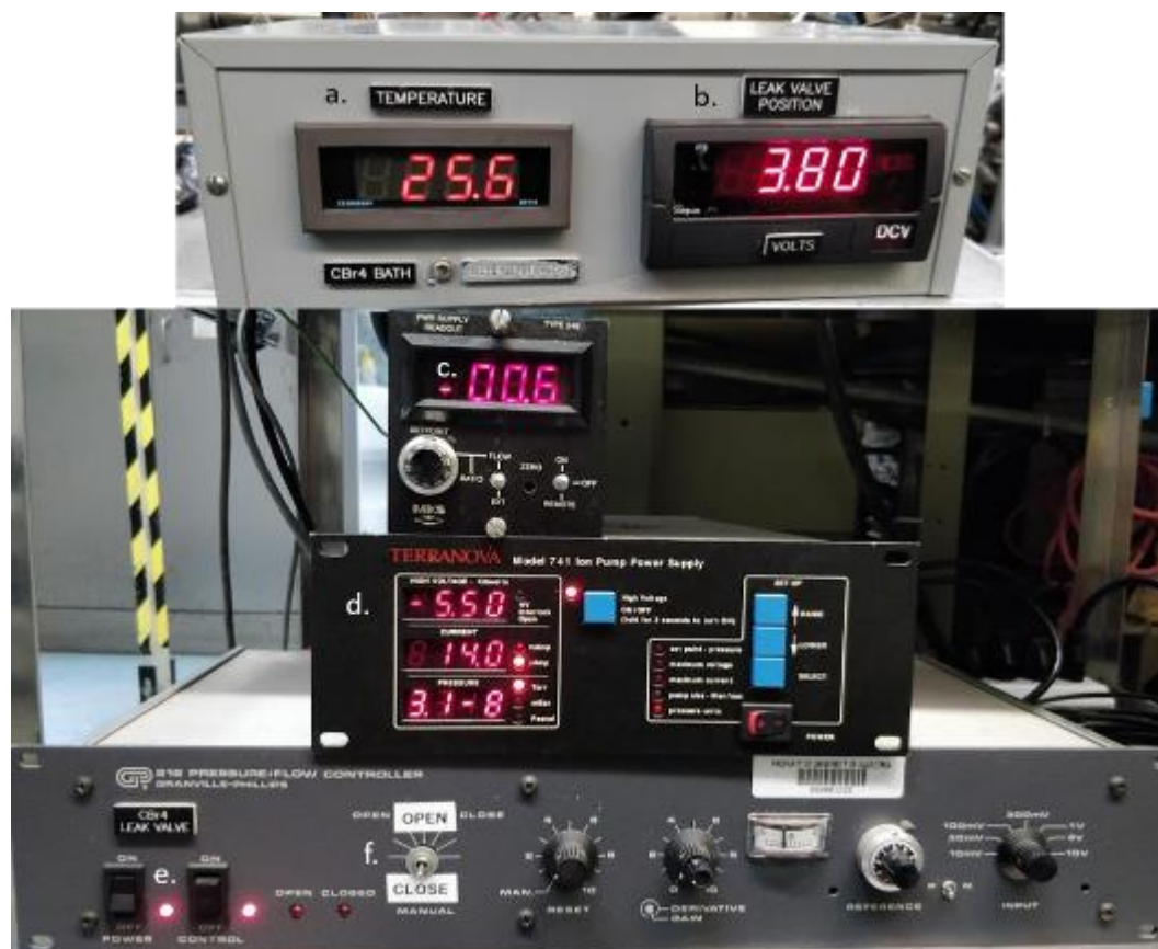
Figure B.3 BBr 3 Control Units on the Cart
