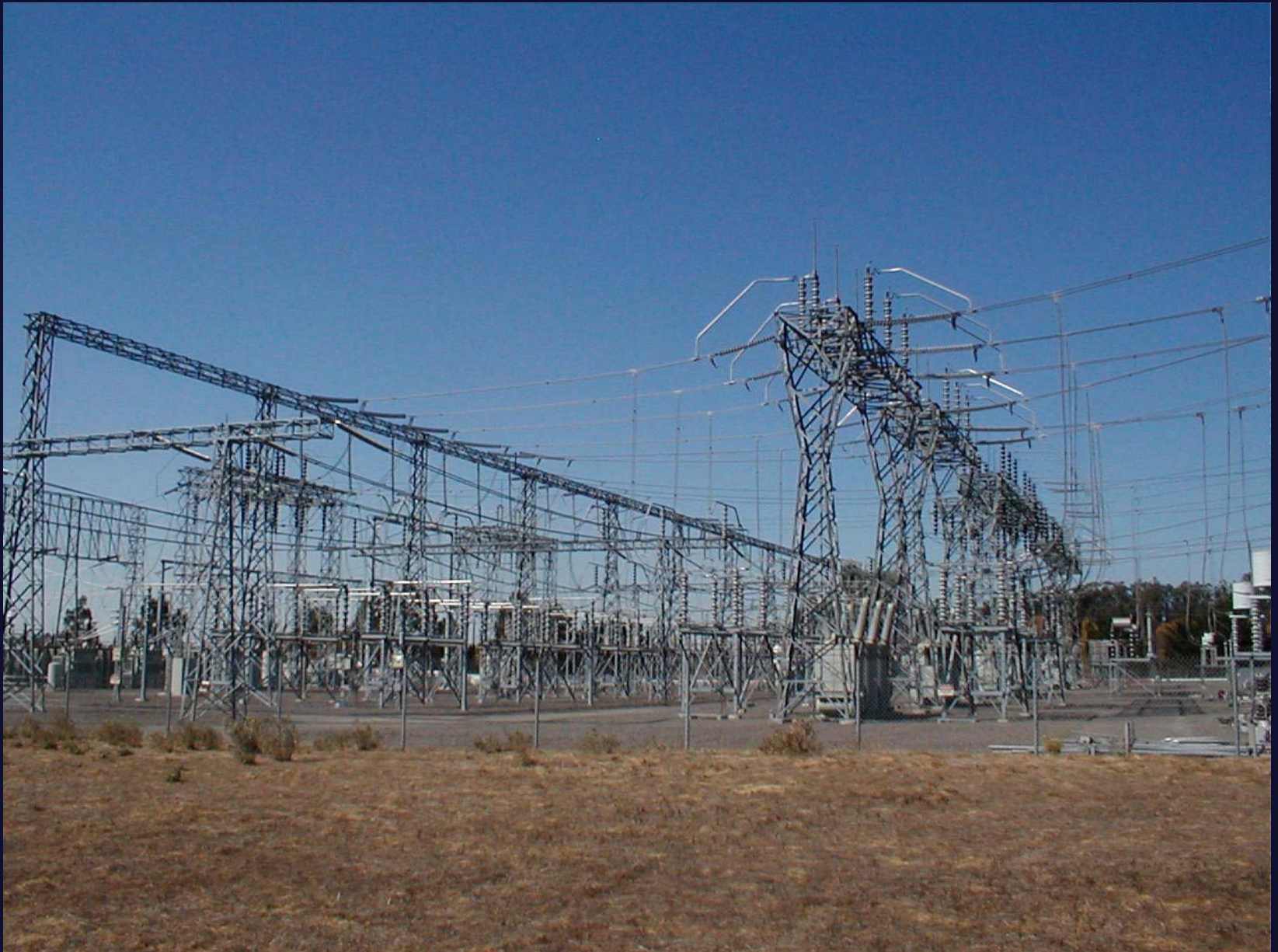
Lakeville transmission substation
