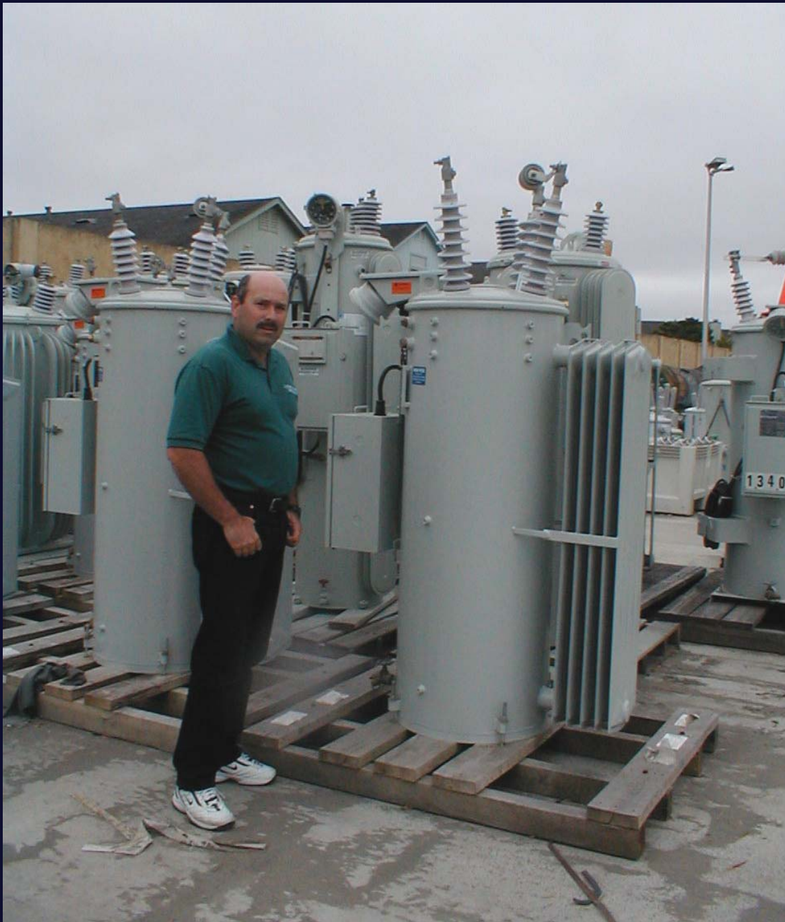
Voltage regulator (on right)
