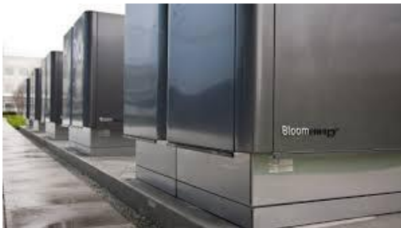
Figure 2: Adobe has installed 12 100 kW Fuel Cells by Bloom Energy on its 5th floor parking garage.
