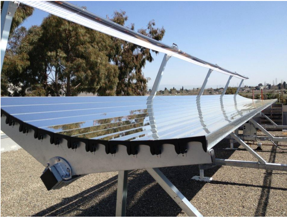
Figure 3. 44-module solar cogeneration system on the roof of one of the cafes. The system has a capacity of 106 kW thermal and 20 kW electrical and will substantially offset the energy required to produce hot water for the cafe.
