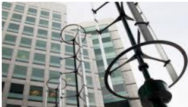
Figure 3: There are 20 vertical axis wind turbines on the 6th floor patio.
