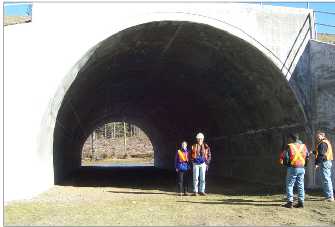
Figure 6. Wildlife underpass designed for elk and deer on the Vancouver Island Highway (1999).
