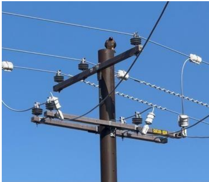
Figure 24. Red-tailed hawk on a power pole. These structures are under-appreciated for their use by large raptors to observe and hunt the landscapes they frequently occur on.
