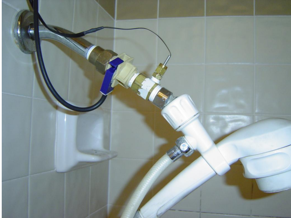
Figure 5. Flow and temperature sensors installed at showerhead.
