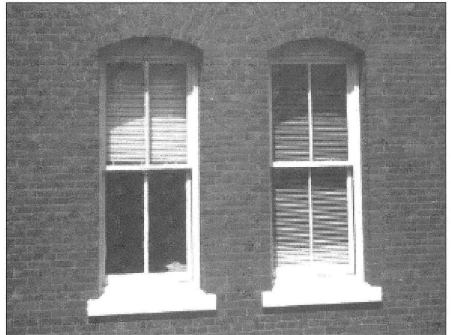
Adjustable interior blinds shade windows and reduce glare without detracting from the historical architecture.
