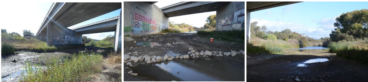
Figure 22. Interrupted flow of surface water.
