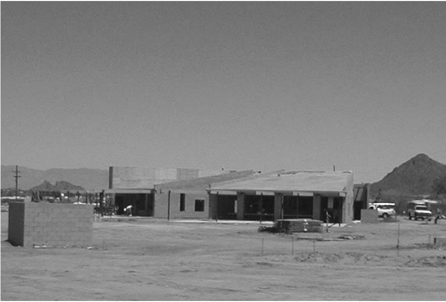
FIGURE 5. A new Head Start facility under construction on the Pascua Yaqui reservation in southern Arizona. Photo by R. Slack.
