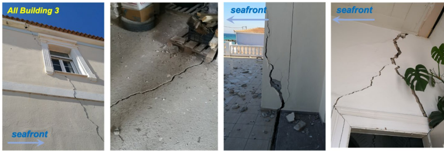
Fig. 17 Building affected by lateral spreading towards the seafront in the neighborhood of Vyrsopepsia in Karlovasi ( 37^{\circ}48'01.1'' N 26^{\circ}42'20.6'' E). The cracks observed running across the building indicate 3-5 cm of movement [photos courtesy of Prof. K. Antonopoulos]
