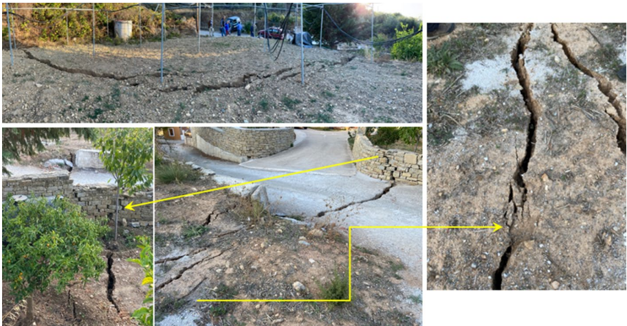
Fig. 24 Ground and pavement cracks in the village of Kontakeika (Samos), indicative of the mobilization of an extended but mild slope or more broadly characterized as seismically-induced secondary ground failures. The cracks extended on both sides of the street through soft soil formations. Arrows in the figure explain the relative location of the cracks
