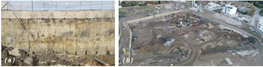
Fig. 25 a Pre-earthquake view of shored deep excavation located in the “new downtown” district in Bayrakli-Bornova ( 37^{\circ}53'50.4'' N 27^{\circ}22'06.2'' E), and b Plan view of the site under discussion
