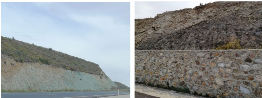
Fig. 19 Selected indicative views of highway cuts with no signs of slope instability ( 38^{\circ}17'31.6'' N 26^{\circ}40'14.6'' E)
