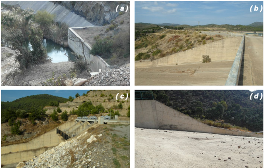
Fig. 29 a Wall on the end of spillway chute of Kavakdere Dam, and side walls of spillways of b Urkmez Dam, c Tahtalı Dam, and d Gumuldur Dam
