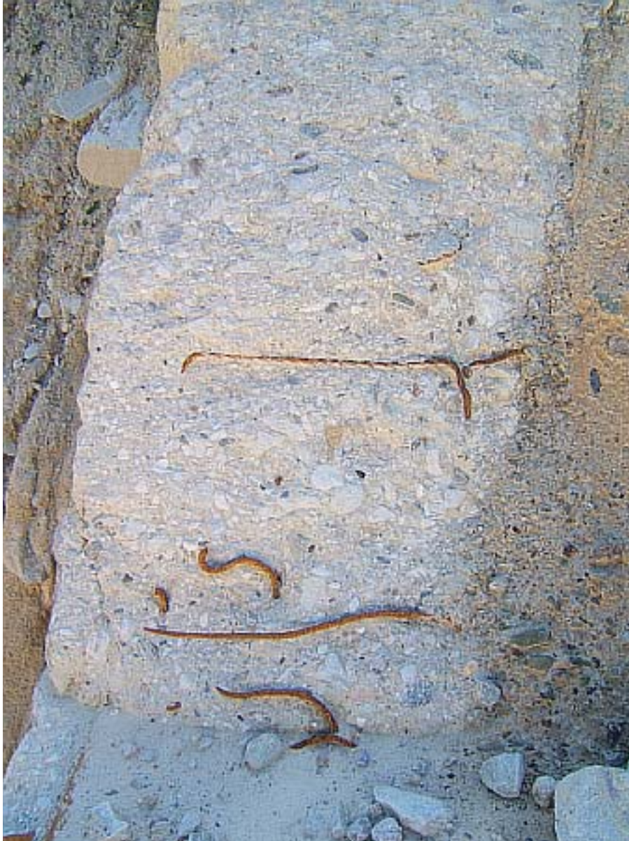
Figure A2. Photograph of the sidewall of a check dam in the Illgraben Torrent, Switzerland. Significant forces on the sidewalls, including those from lateral accelerations at the front of boulder-rich snouts, caused erosion on the order of centimeters, exposing the steel reinforcement. The width of the dam is \sim 1 meter.
