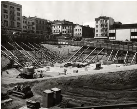
Figure 23: 1961 - The construction of the Portsmouth Square parking garage required fully excavating the existing square.
