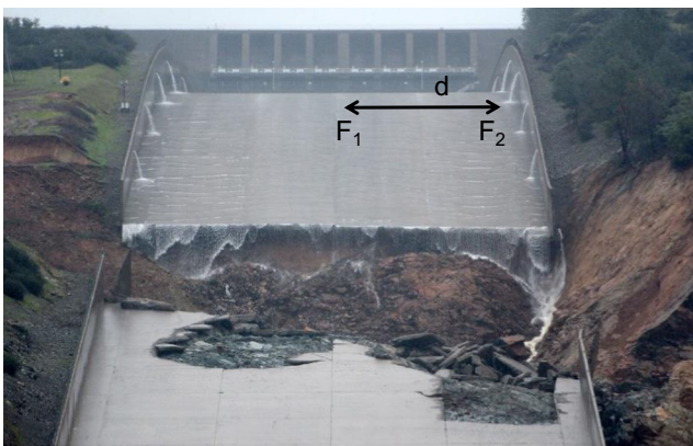
Fig. 1 Photo of a collapsed spillway of the Oroville dam
