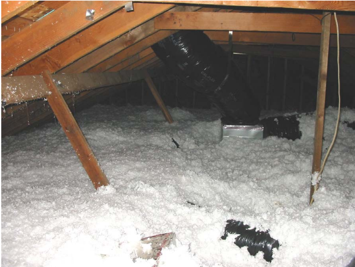
Figure 4. New flex ducts in attic covered by additional blown-in insulation after the retrofit.
