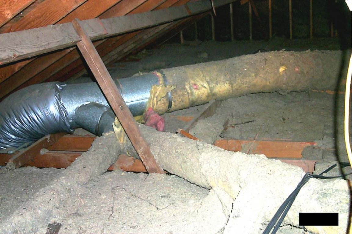
Figure 3. Poorly insulated sheet metal ducts and blown-in insulation in the attic before retrofit
