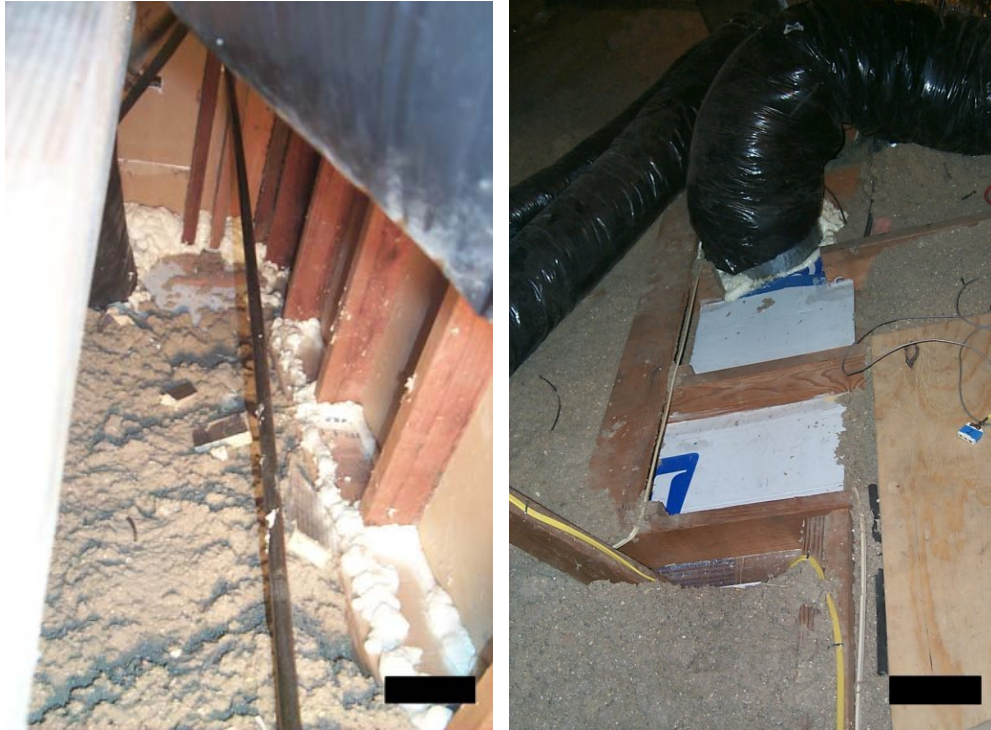
Figure 1. Sealing cavities connecting the house to the attic. Foam was used for sealing small holes and cracks at building component intersections (left). Duct board insulation was used to block off large open areas (right)
