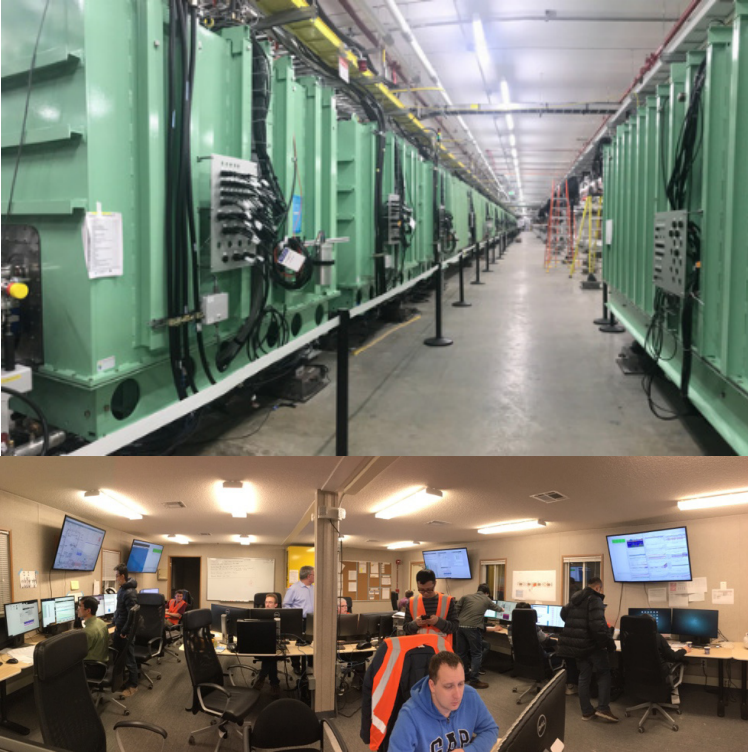
Fig. 6. ARR3 beam commissioning in 2019 including the front end, 15 cryomodules of both \beta = 0.041 and 0.085 QWR of FRIB linac segment 1 (LS1) and part of the FRIB folding segment 1. (Top) View inside the FRIB accelerator tunnel with 15 commissioned QWR cryomodules of linac segment 1 to the left and \beta = 0.53 half-wave resonator (HWR) cryomodule of linac segment 3 to the right. (Bottom) The ARR3 commissioning team at the FRIB main control room.
