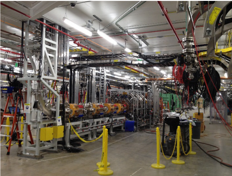
Fig. 1. FRIB driver linac viewed from the lower low-energy-beam-transport (LEBT) towards the superconducting linac in the accelerator tunnel at the beginning of beam commissioning in 2017.
