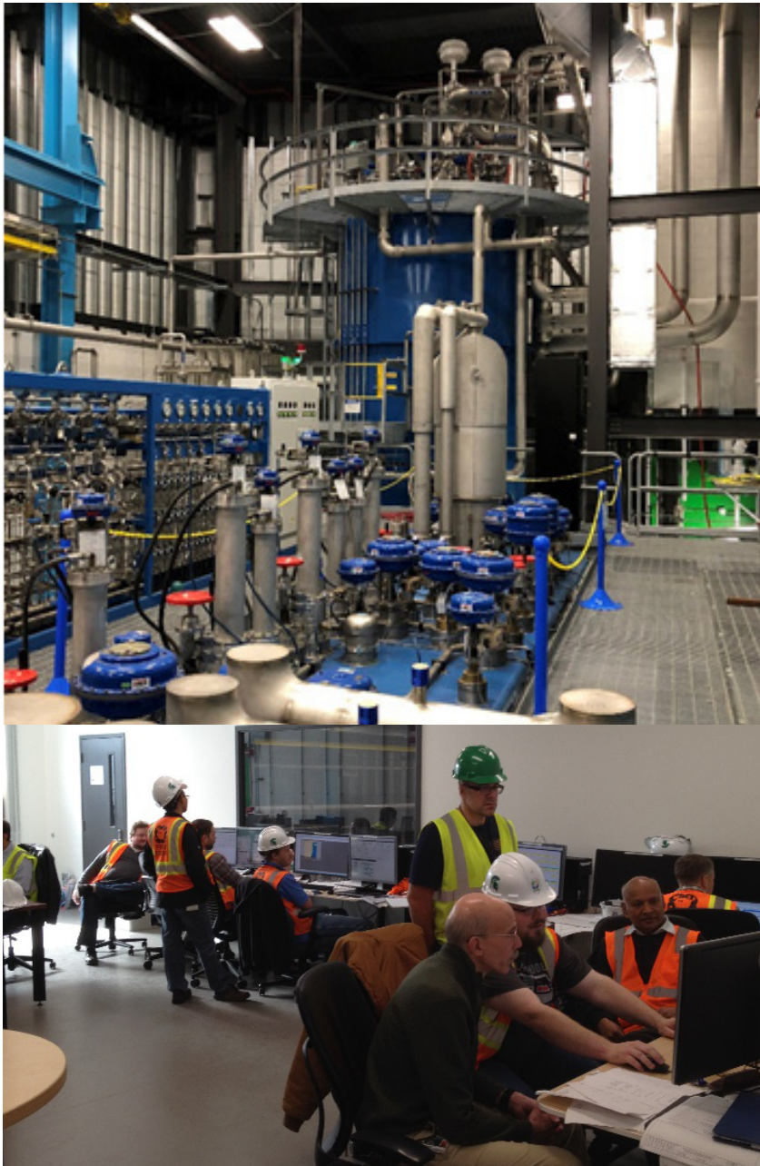
Fig. 4. Commissioning of the FRIB helium refrigeration system (cryoplant) at 4 K in 2017. (Top) The FRIB cryoplant established to supply liquid helium to the entire FRIB accelerator facility. (Bottom) The FRIB cryogenics team during the cryoplant 4 K commissioning in the FRIB cryogenic control room.
