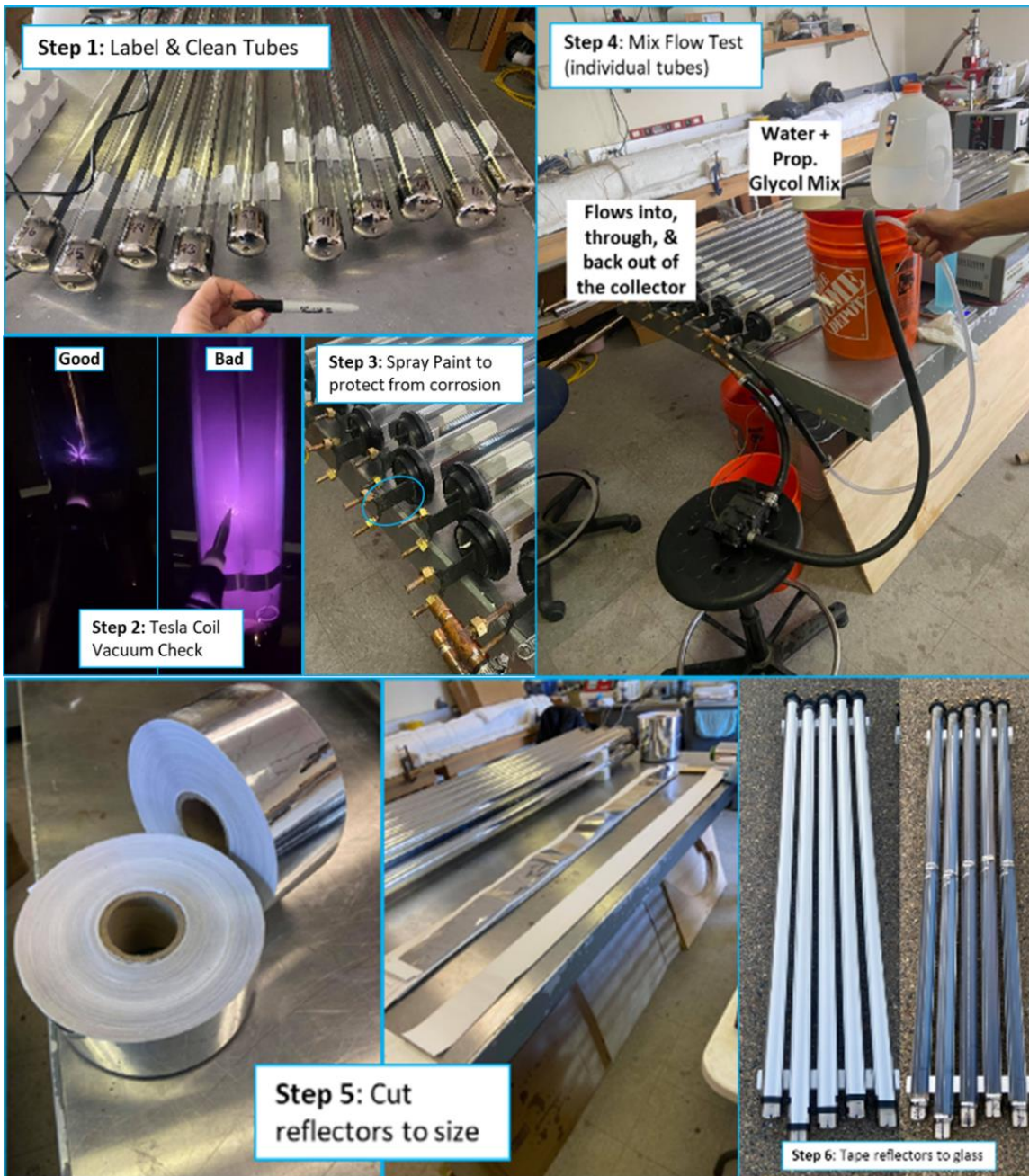
Figure 43: Outline of steps for individual tube inspection and reflector application
