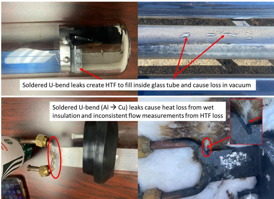
Figure 52: Leak points on the current ICPC design
