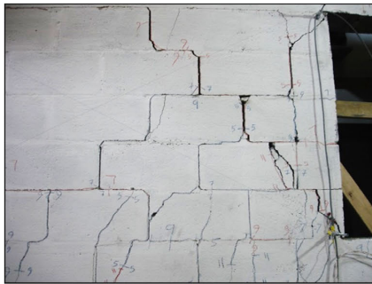
Damage in left pier
