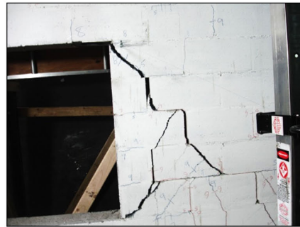
Damage in right pier
