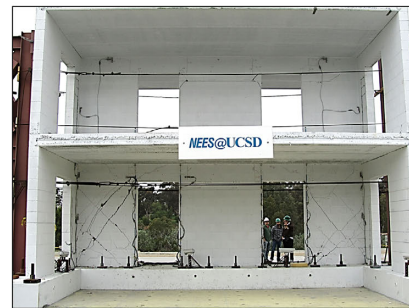
(b) Shear cracks in first-story walls after the tests
