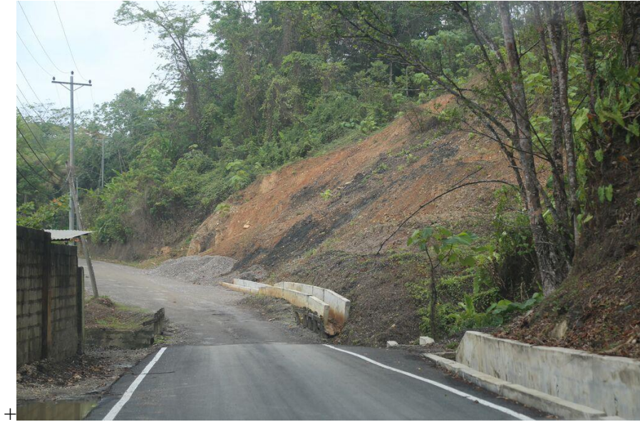
Figure 9. Exposed hillside which is susceptible to sliding during rainy periods
