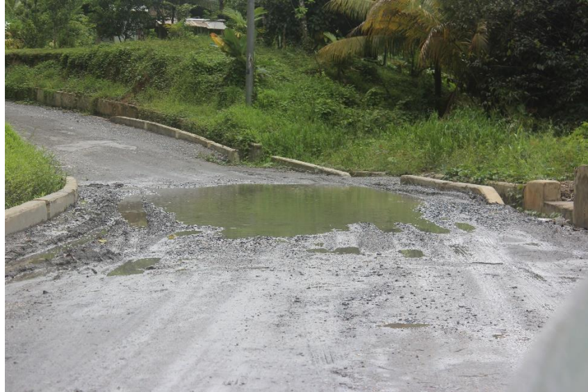
Figure 18. Large hole in road in Matelot filled after rain event
