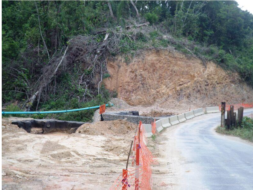
Figure 11. Exposed vertical slope where landslide previously occurred
