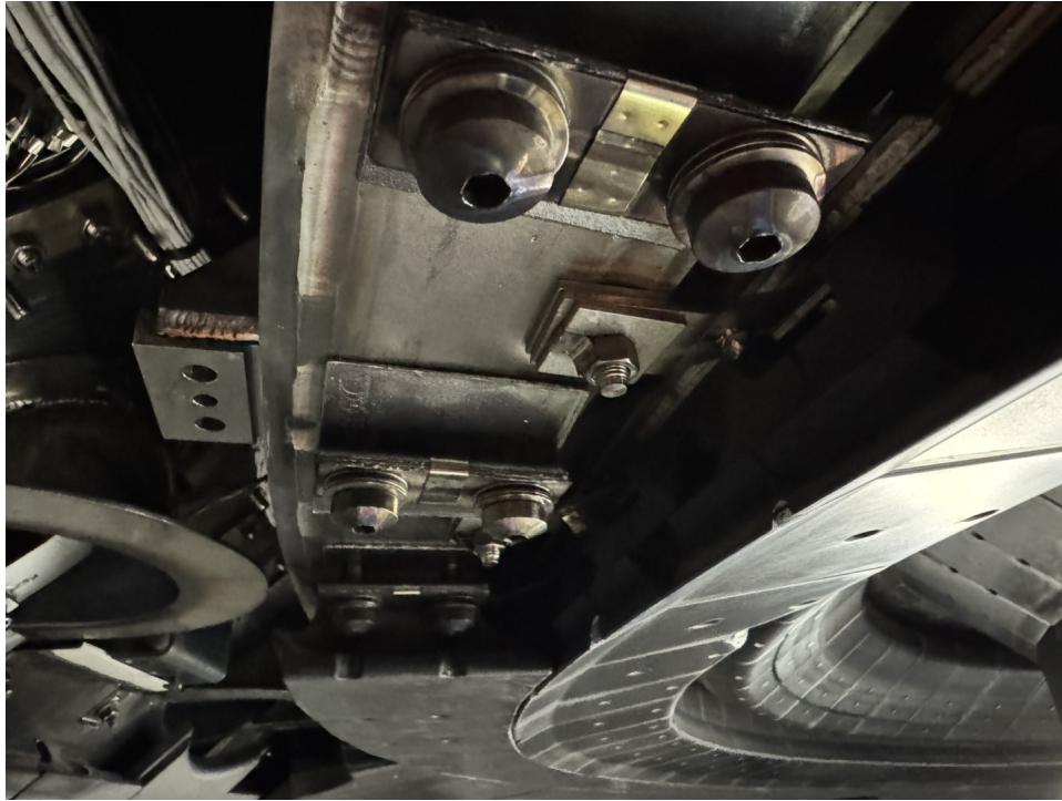
Figure 2.11: Standard nut bars used for mounting tiles in the DIII-D vessel. Image depicts nut bars installed on the water-cooled plate in row B (see 2.1.2), with tiles uninstalled.
