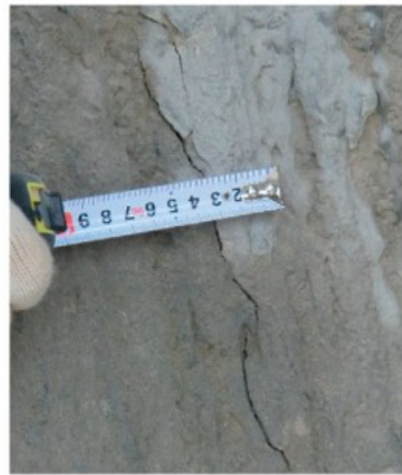
(b) Crack B on the cut slope.
