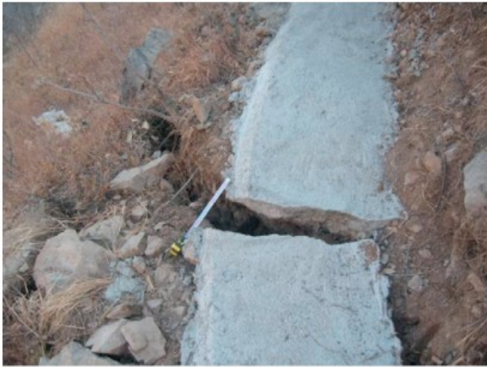
(a) Crack A on the natural slope.
