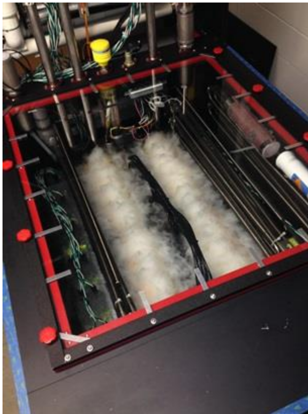
Figure 5-2: Pilot Test - IT Running at Full Power.
