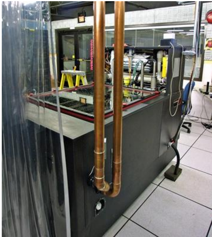
Figure 5-3: Immersion Case Test Installation (Demonstration)
