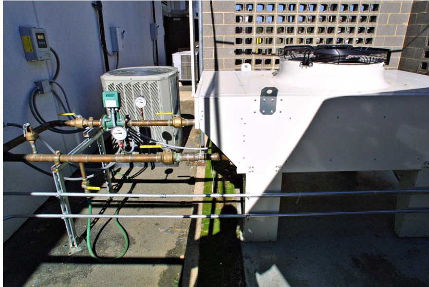
Figure 4-3: Dry Cooler Outside of NRL Data Center
