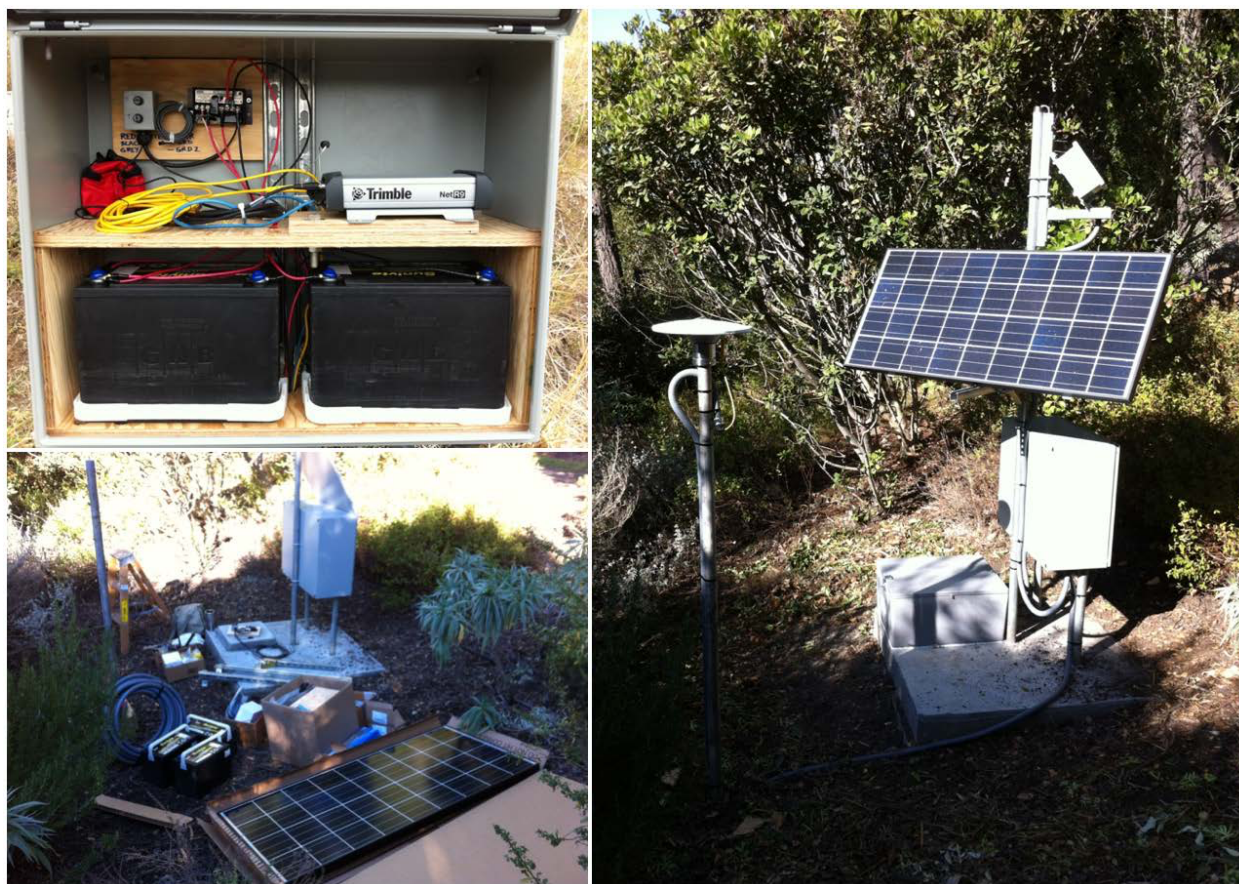
Figure 5-5. cGPS station equipment and setup at LRA6.
