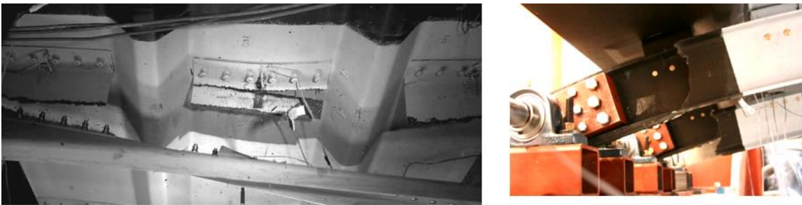
Figure 4.2: Combined bending-twisting failure in C-frames [8,11].
