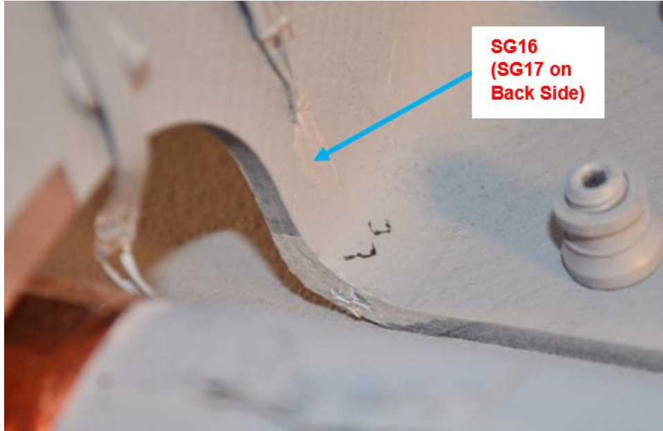
Figure 3.83: Paint chipping observed on Loc3 shear tie radius after Loc3-1_L1.
