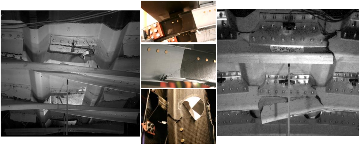
Figure 1.4: Severe internal damage by HEWABI (shear tie and C-frame fracture) [8].
