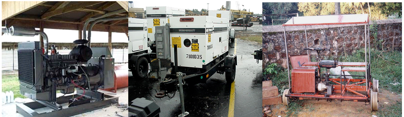
Figure 5 Left, diesel-electric generator providing local electric power for a small community. Center, typical mobile diesel-electric generator for backup and emergency power. Right, diesel-electric generator fabricated from an old railroad utility cart. (Google Images: http://images.google.com/ )
