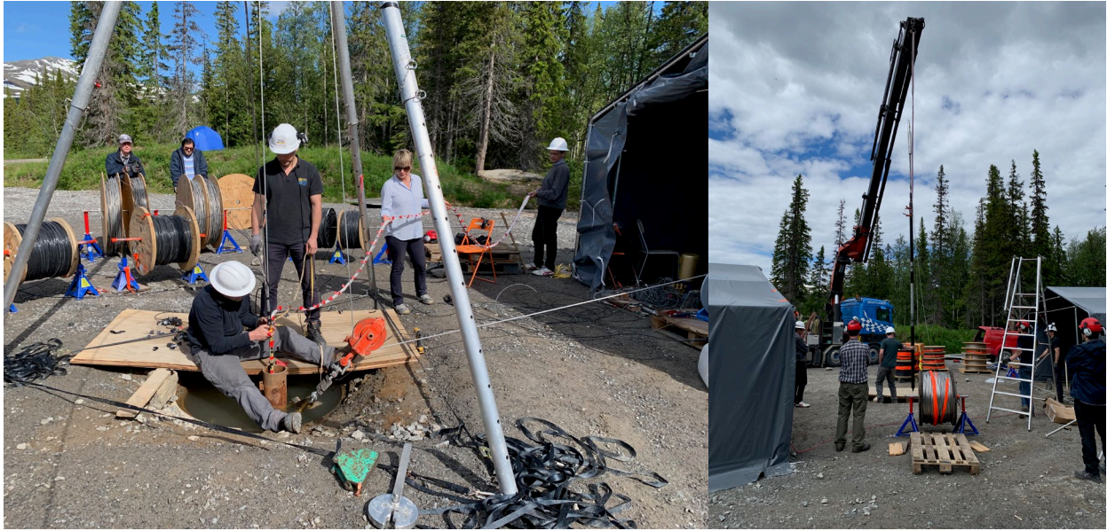
(Left) – Detaching the SIMFIP conductivity strip from the wireline. (Right) – Pulling the SIMFIP tool out of the borehole.
