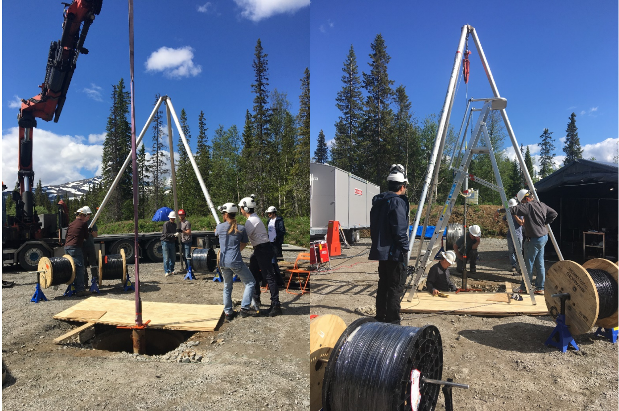
(Left) Moving the tripod into place (Right) Securing the bottom sheave onto the wellhead.
