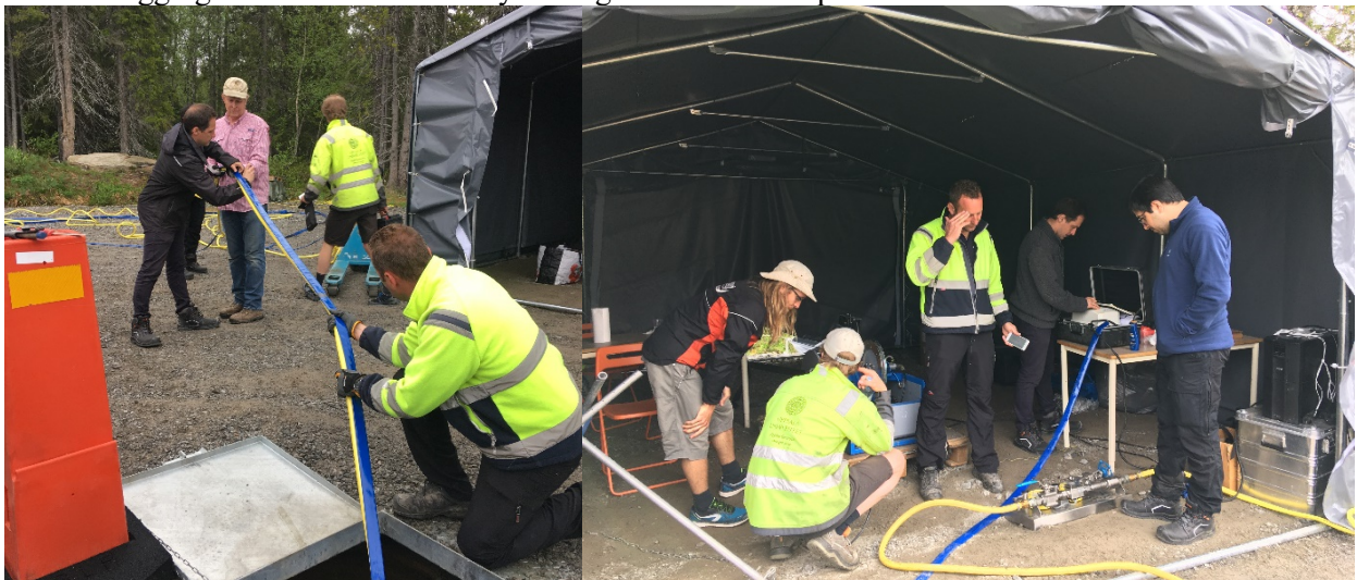
Deployment of downhole pump to lower head for FFEC logging run the next day.
