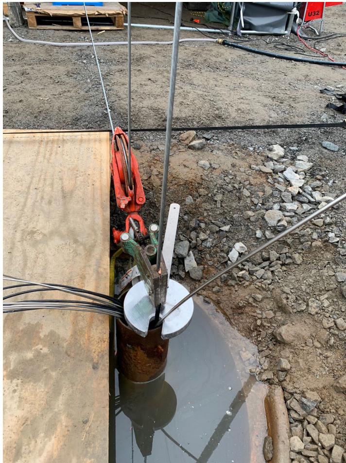
The wireline clamp and "frying pan" tool in place securing the line from moving downward after the wireline "free fall" event.
