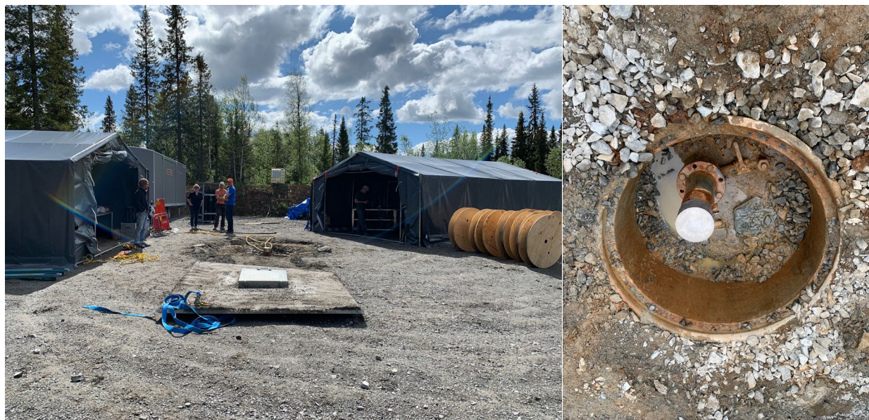
(Left) Removal of the metal wellhead cover so that we could directly access the wellhead (Right) Bailed out wellhead – open bolt holes can be used to secure the bottom sheave.
