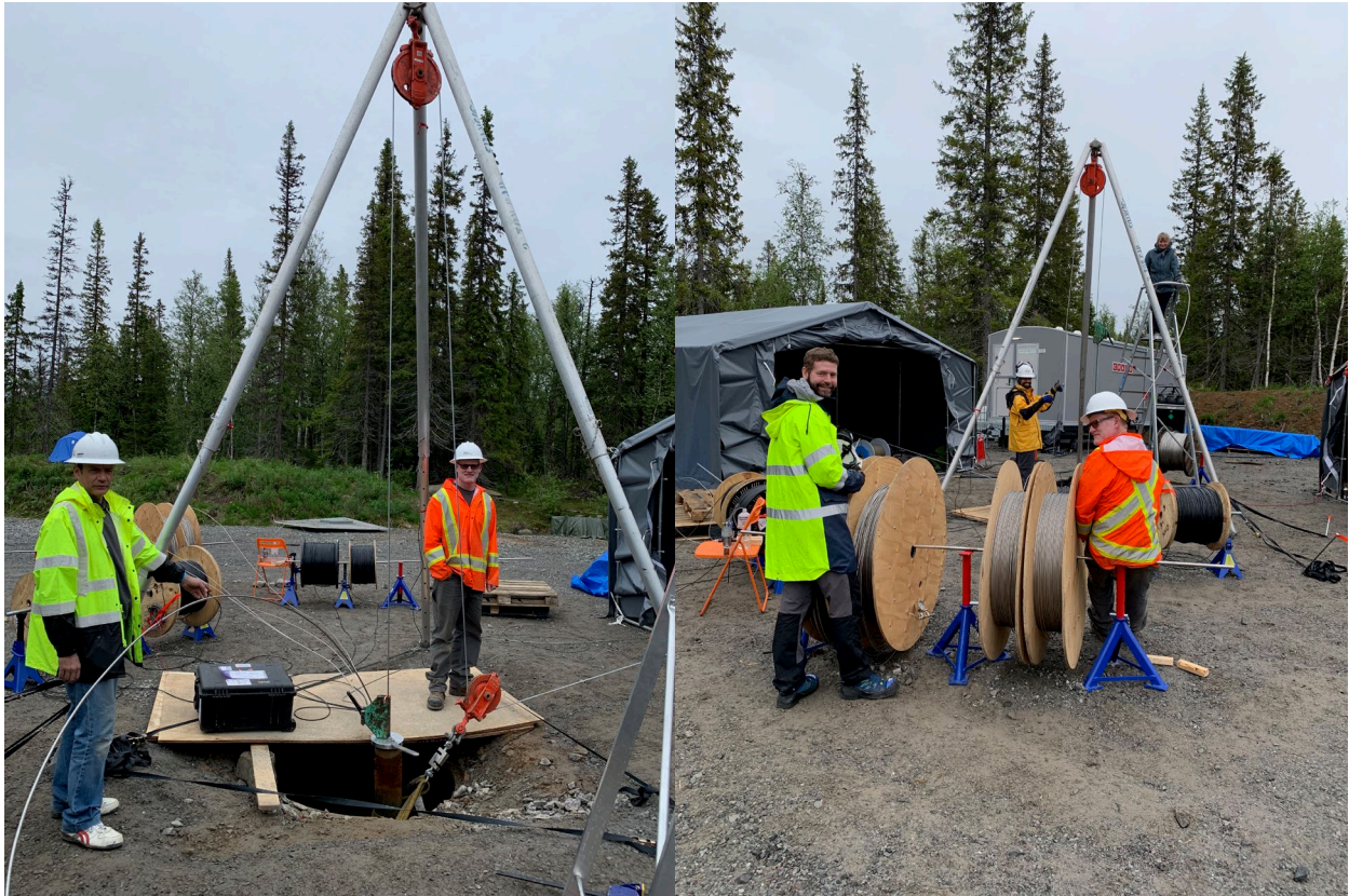
(Left) Successful rerigging of the load cell onto the lower sheave. Note wireline clamp and “frying pan” in place. (Right) Auli overseeing our operations from above!
