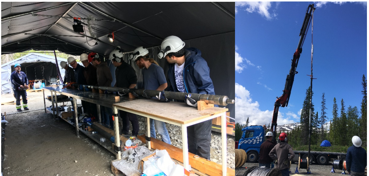
(Left) The team lifting the SIMFIP tool off of the table (Right) The crane lifting it in the air prior to positioning it partway into the borehole.
