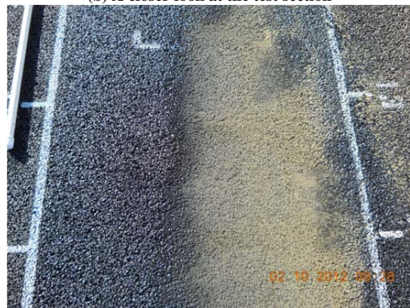
(d) Signs of subgrade rutting and crack initiation near Station 13 but no moisture damage in the asphalt
