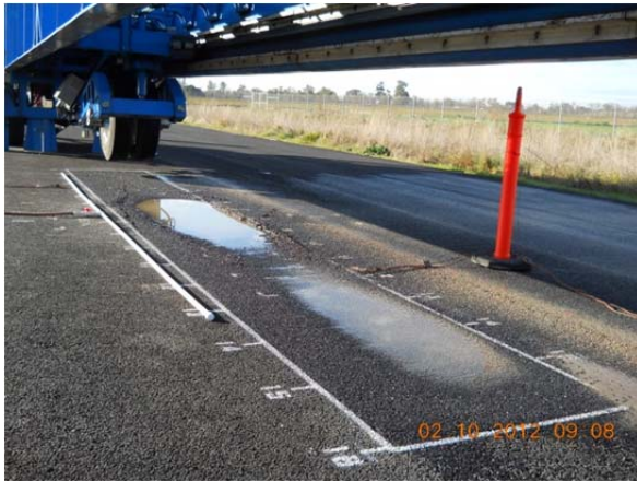
(a) Overall view of the failed pavement
