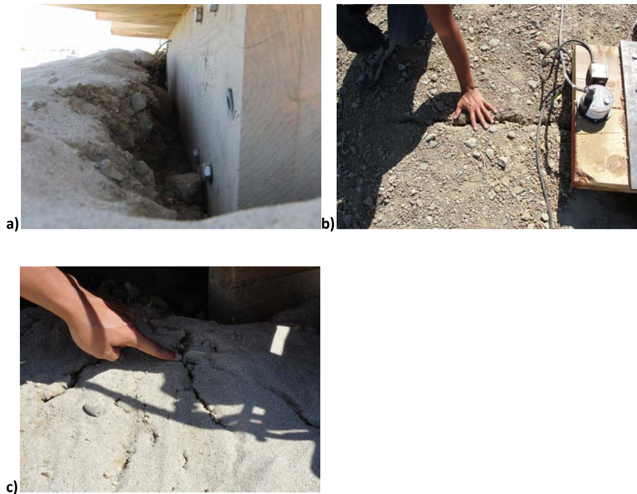
Figure 4.20: Damage to the model levee after August 2011 tests: a)Gap formation between timber shaker base and soil, b) 1m long crack on left side of embankment crest, c) 0.3 long cracks on right side of embankment crest
