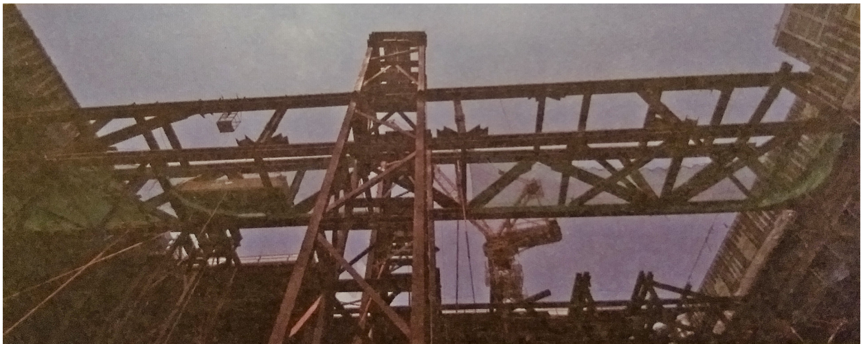
Figure 20. The "mega-truss" that enables the "unobstructed communication of grace." This photo, which was shot from a perspective that gives the mega-truss a visual similarity to a cross, is featured in Sarang Church's book about the building project.
