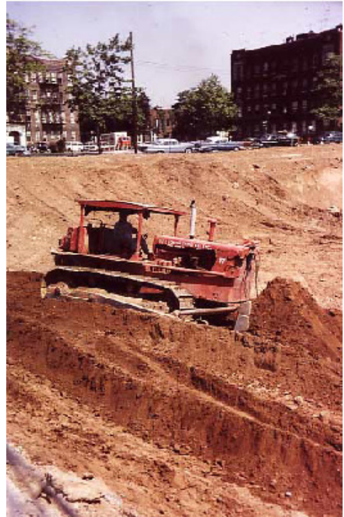
Figure 10. A Gull Contracting Co. vehicle shovels earth in Bay Ridge to make way for the Verrazano-Narrows Bridge. Source: Walsh 2003
