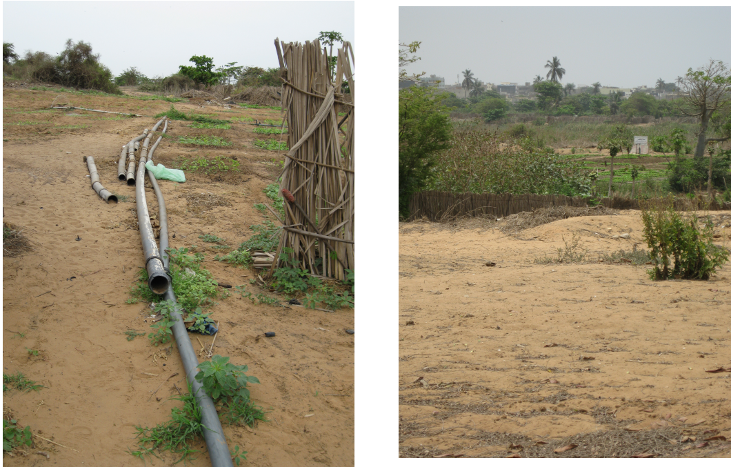
Figure 17: Photographs of Pikine’s wastewater treatment projects (Source: Author)
