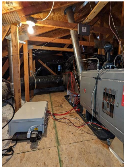
Figure 10. Data acquisition enclosure in attic of Site 2
