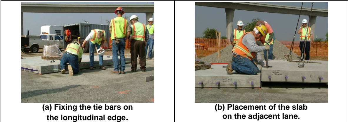
Figure 8. Fixing the tie bars and placement of the slab on the adjacent lane.
