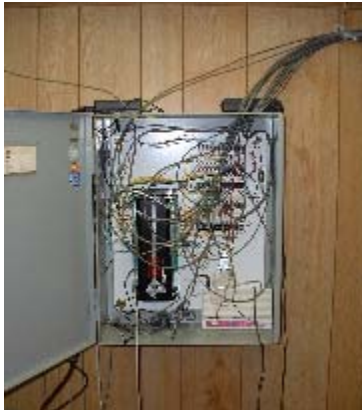
Figure 34. Kaprielian Brothers Packing Company (Cold Storage) Facility in Reedley: Data logger box.
