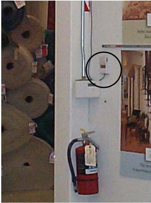
Figure 6. Carpeteria Flooring Center in Sacramento: Indoor air temperature sensor.
