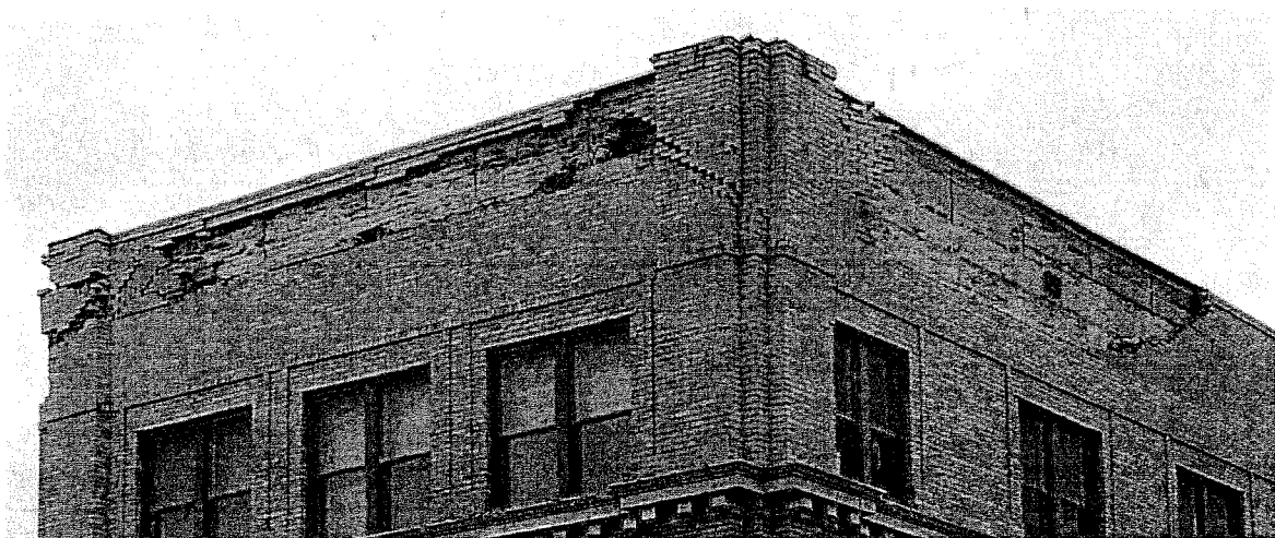
Figure 23: Separation of the outer wythe in the parapet of a historic URM building. December 22, 2003 San Simeon, California earthquake ( http://peer.berkeley.edu/san_simeonEQ/ ).
