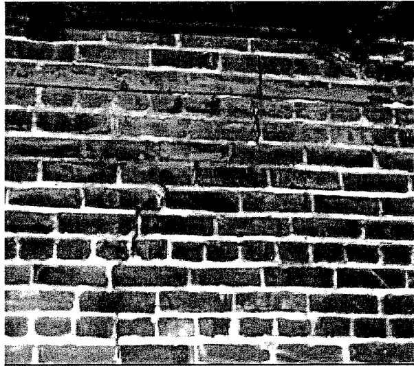
Figure 5: A typical historic URM building with in-plane shear cracking in a multi-wythe load bearing wall. December 22, 2003 San Simeon, California earthquake ( http://peer.berkeley.edu/san_simeonEQ/ ).
