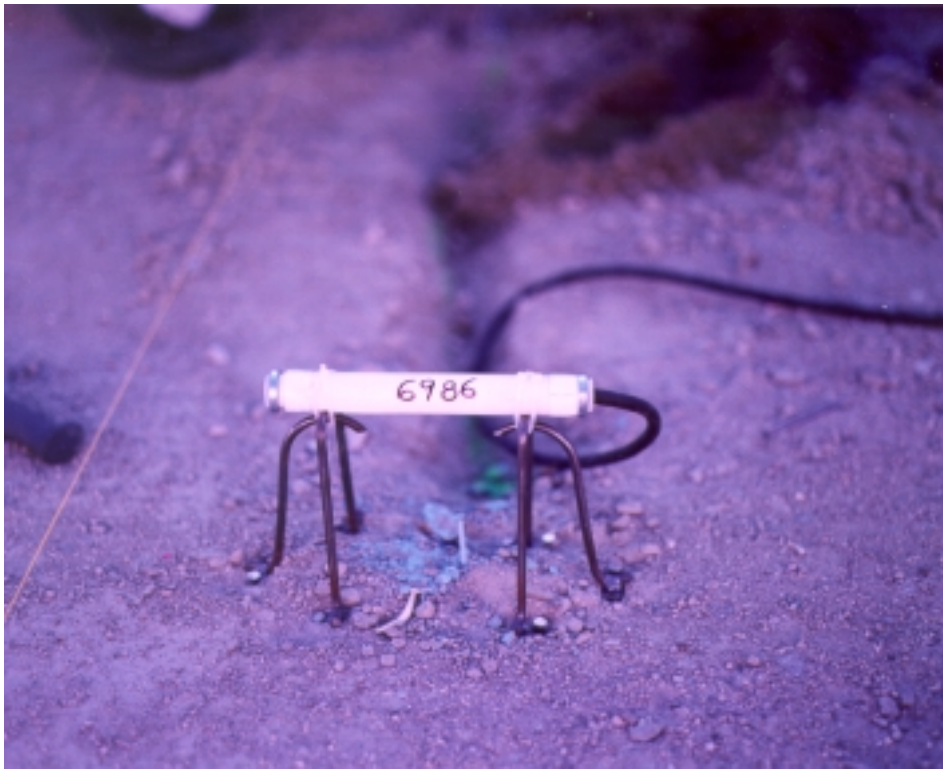
Figure 6.4. Steel Frame with Carlson A-8 Strain Meter Installed on South Tangent.
