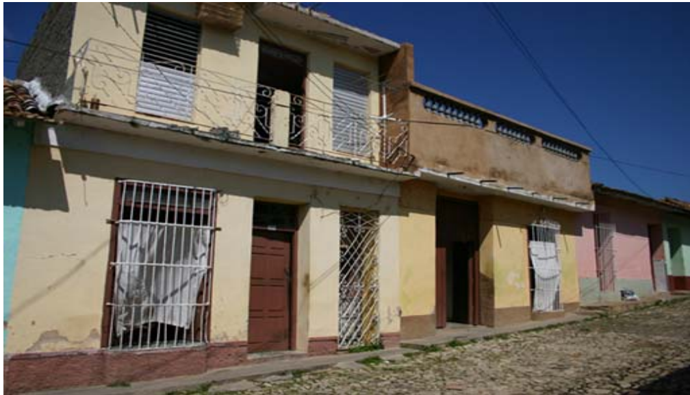
Figure 2.2 “Contamination”: Restoration in violation of the building code. Photo by Maki Tanaka.
