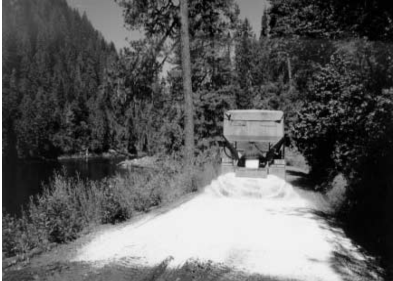
Fig. 5. Calibrated spreader applying Calcium Chloride to a previously processed road. The result is a finished road with a hard, smooth, maintainable driving surface. Grinding with the In Place Processor also works well in frozen soil, as the rocks stay in place for crushing. Some dampness in the soil is preferred for decreased machinewear, dust control, and compaction.
