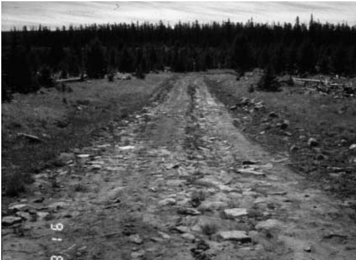
Fig 1. Typical example of a worn-out, un-maintainable road.
