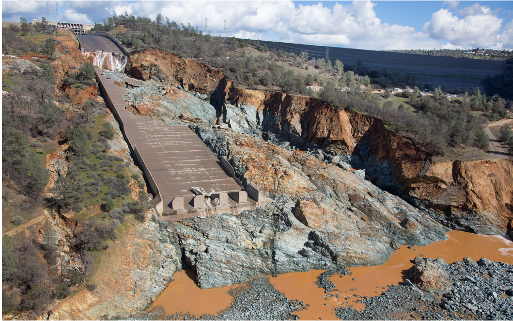
Figure 1.2: Scour damage to service spillway at Oroville Dam in Northern California, 26 February 2017 [58]
