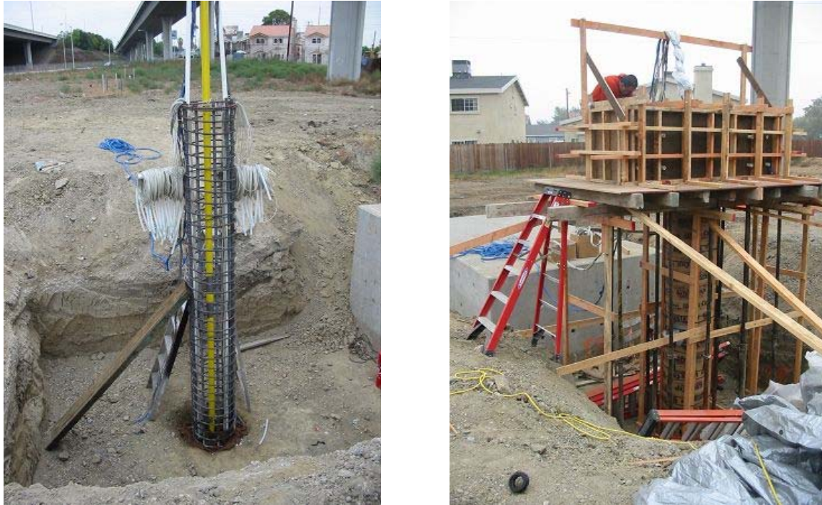
(a) (b) Figure 2.6. Construction of (a) shaft below grade and (b) shaft and cap above grade.
