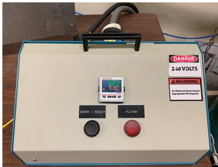
Figure 17. Heater Controller Box
