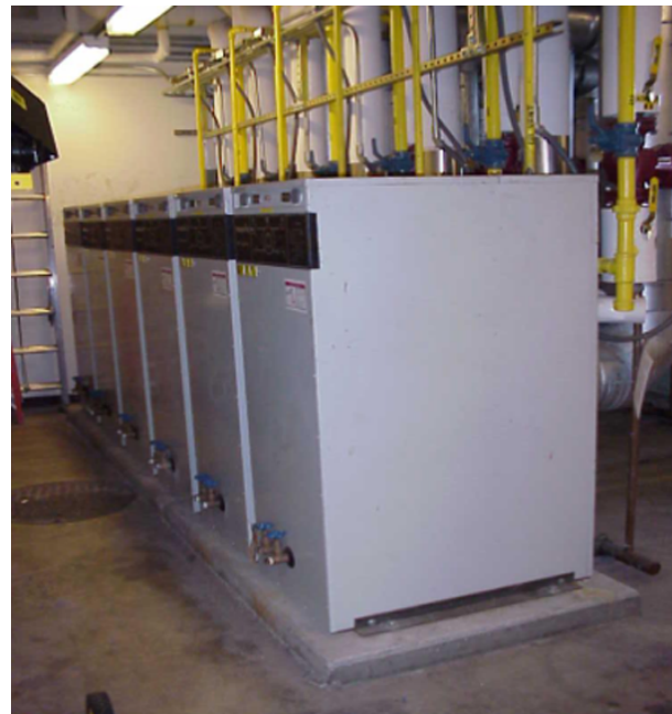
Figure 4. LBNL replaced two boilers with 11 modular boilers to maximize part-load efficiency.
