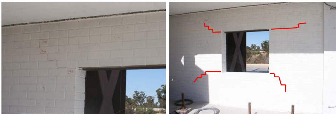
(a) stair-crack at window corner
