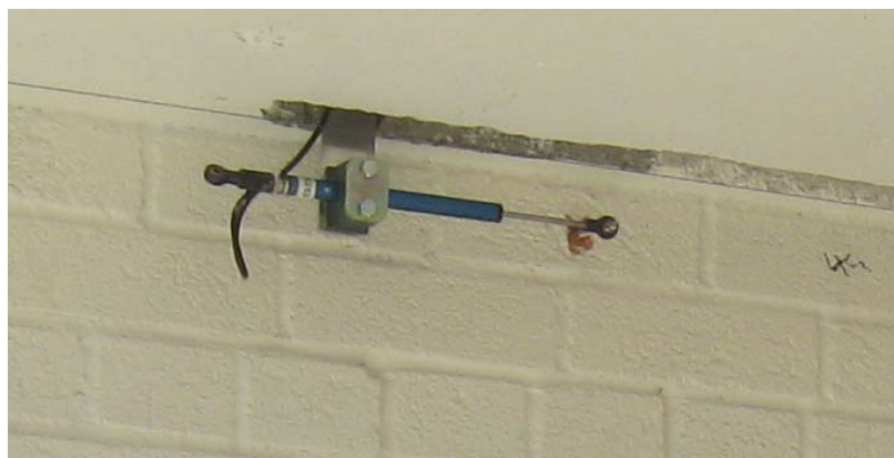
Figure D.7: LVDT measuring the sliding of the infill wall with respect to the beam.
