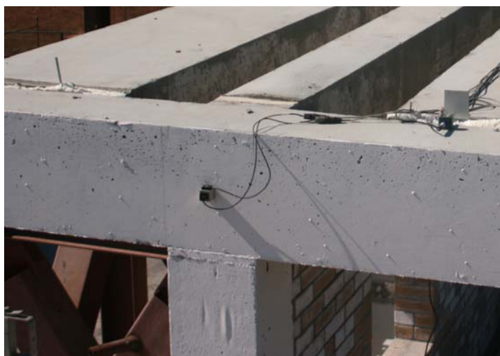
Figure D.5: Accelerometers at east end of the structure at the roof level.
