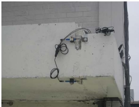
Figure D.1: LVDTs used to measure the rotation of slab-to-beam hinge connection at the first story.
