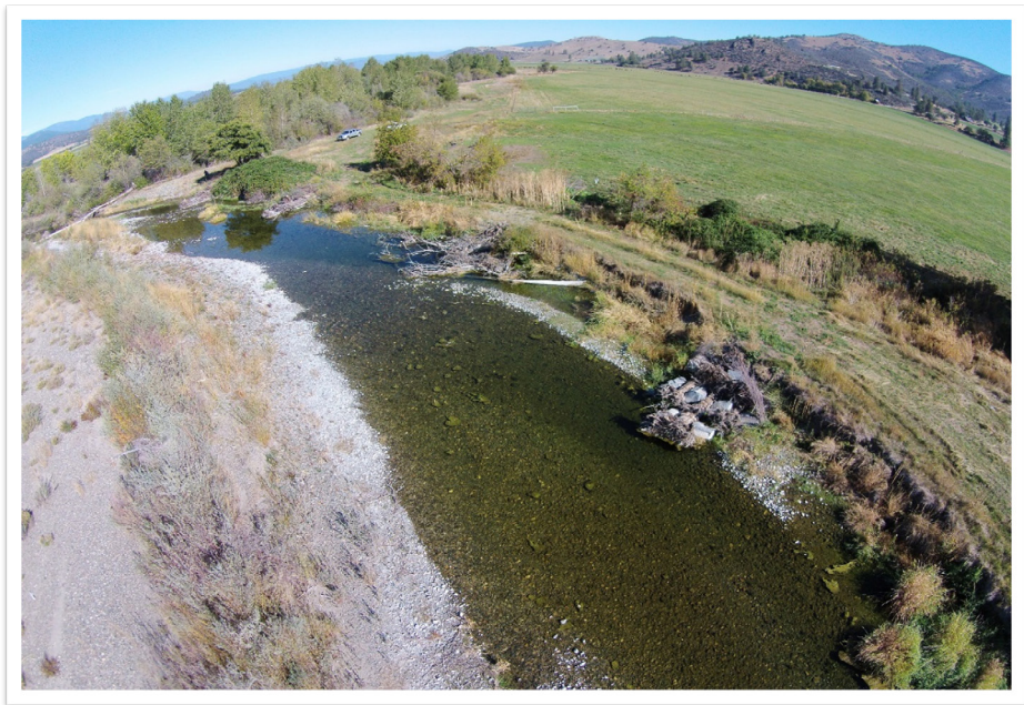
Figure 10. Large wood structures redirecting the flow from an eroding streambank. Photo credit: Joey Howard, Cascade Stream Solutions.
