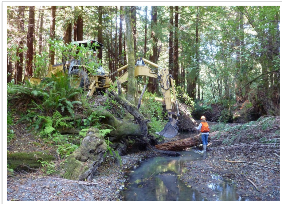
Figure 16. Log being positioned with a rubber-tired backhoe. Photo credit: Derek Acomb, CDFW.
