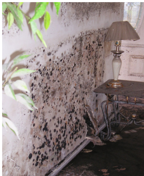
FIGURE 24.6.1 Mold growing in a flooded home after Hurricane Katrina, New Orleans, 2005. Photograph by Gina Solomon.
