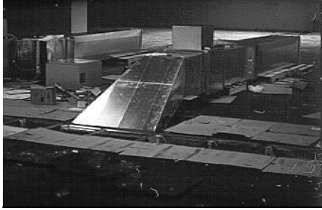
FIGURE 5 Photo of supply fan and inlet duct at CBE Underfloor Air Supply Plenum Test Facility
