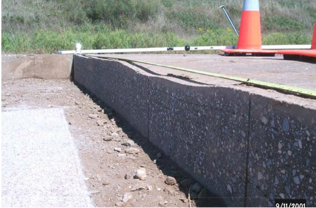
Figure 3.3: Photograph of the cross section of rutted HMA layer in trench in Cell 21 after trafficking.
